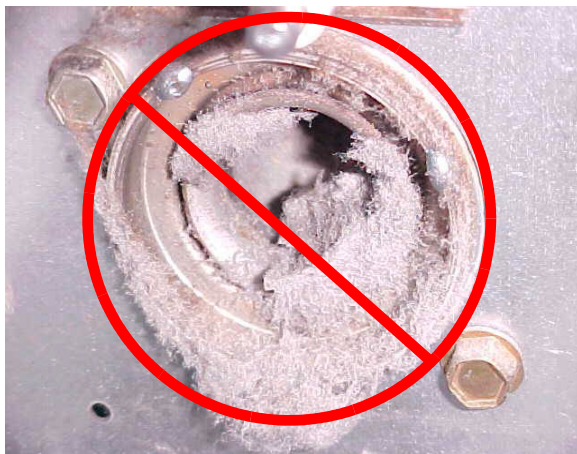
Burner Tube with Lint Buildup
